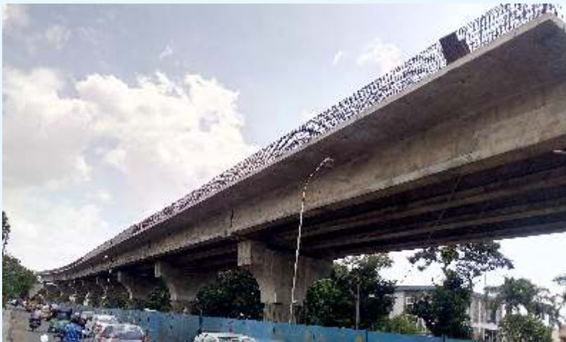
Ongoing works of Grade Separator at Pallavaram Junction on GST Road in Chennai
