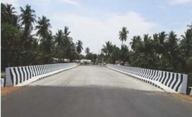
Bridge at Jedarpalayam in Namakkal District (Inaugurated by Hon'ble Chief Minister on 08.05.2017)
